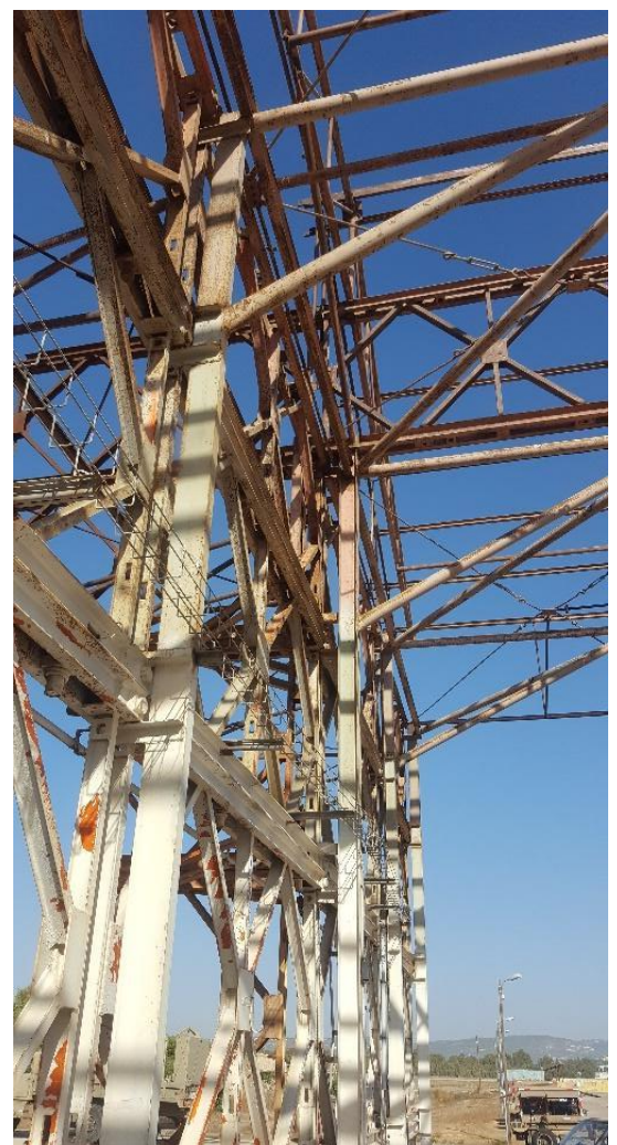
shed condition before treatment
