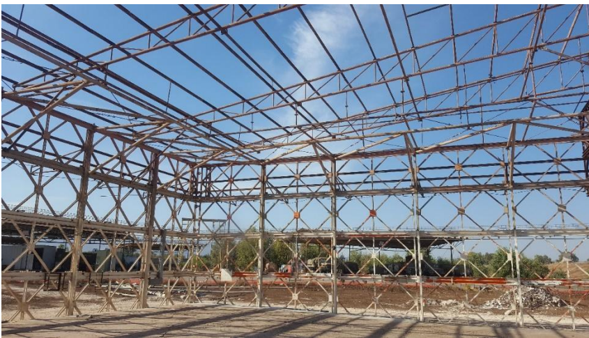
shed condition before treatment
